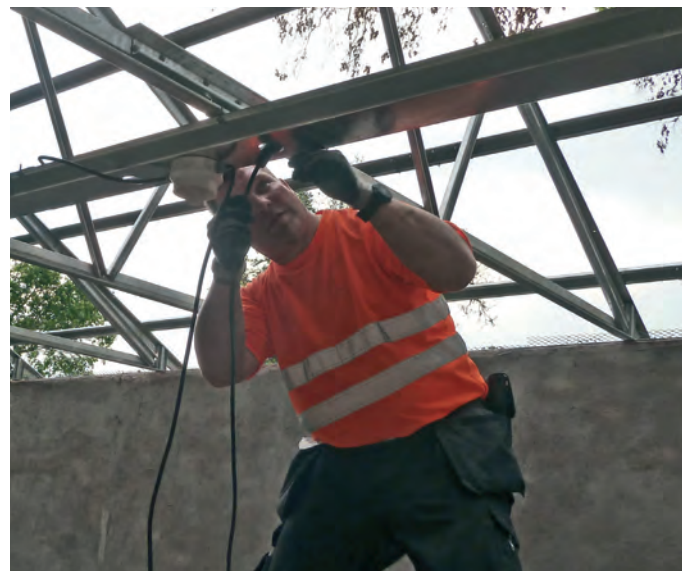
Earth House's electrical installer Timo Kettunen building a grain storage unit commissioned by Irish Aid in Zambia's North Territory, north of Luwingu. "This unit was the first in which we used Ensto's electricity. Ensto's solution streamlined the installation, and sped it up by at least three days in difficult circumstances - not to mention the quality!"
