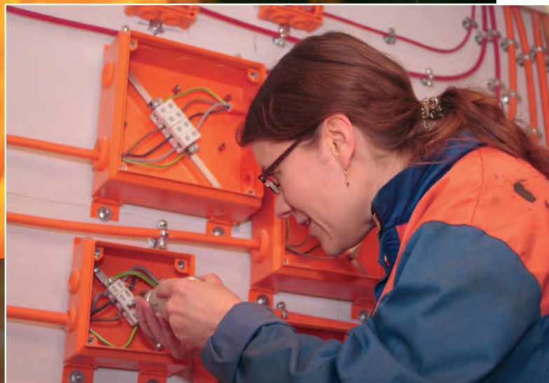
Ensto Product Manager Riitta Seeck prepares Ensto Vulcano for its trial by fire.
